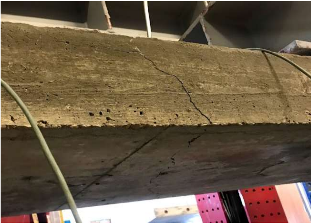
Figure 5-24 The wide crack that propagated on UBS2 beneath the loading beam (top) and the fine crack that propagated on UBS2 at almost mid-span (bottom)
