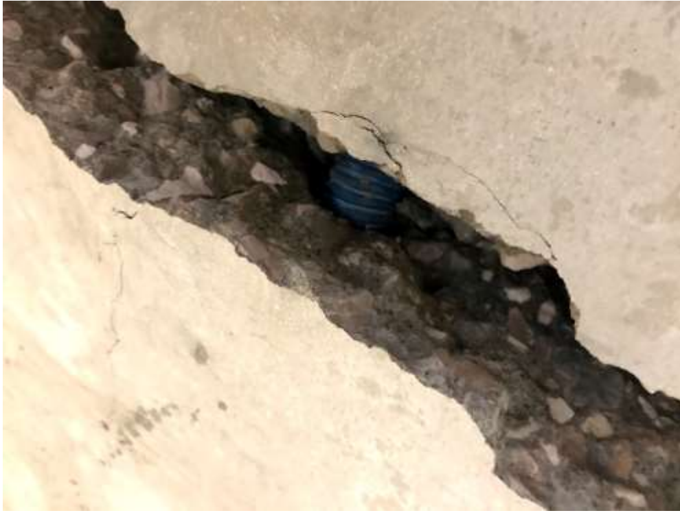
Figure 5-3 BS1 wide crack at failure viewing an unbroken tendon
