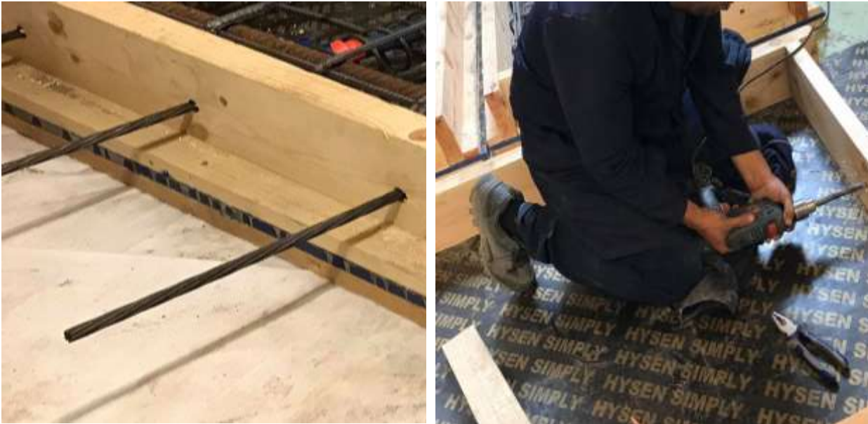
Figure 4-6 The bonded tendons pointing out of the slab specimen edge with length 30 cm (left) and drilling the holes (right)
