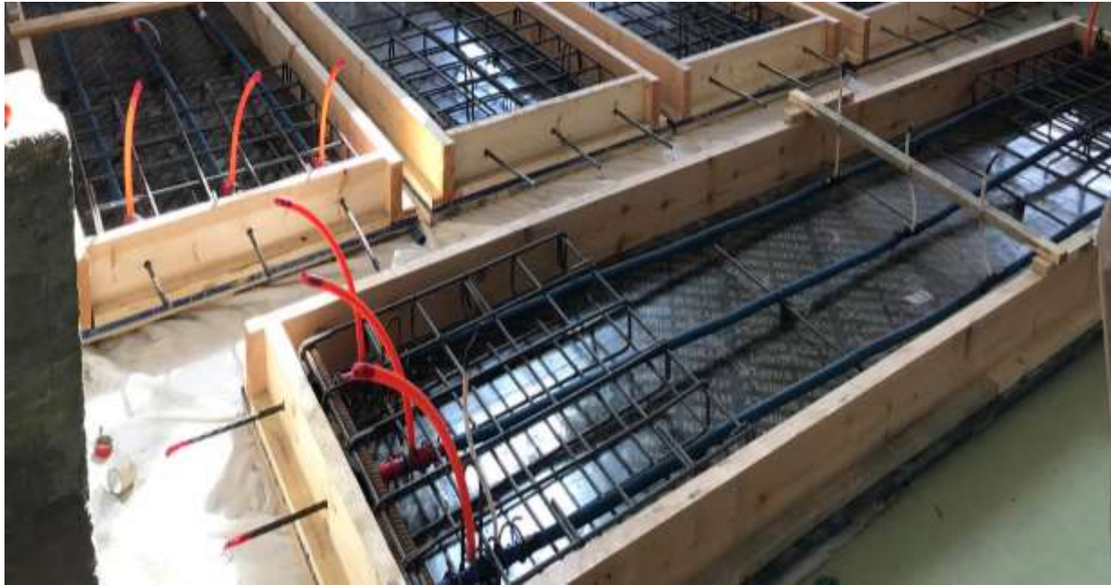
Figure 4-9 The full setup of the BS1 after installment showing the designed tendon profile installed using chairs and steel bars
