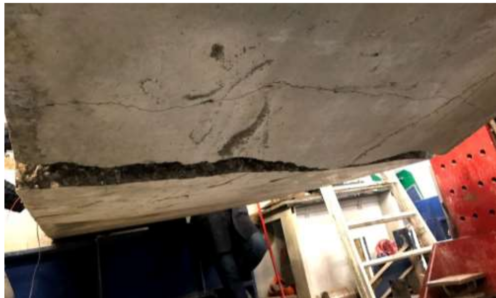
Figure 5-2 BS1 after failure (top) and formed cracks after failure in a view from the slab's soffit (bottom)
