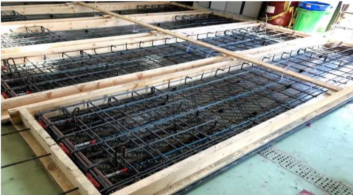
Figure 4-12 The slab specimens after the installment of all of the elements and the supporting wood panels attached to them the plastic tubes containing the strain gauge's wires.
