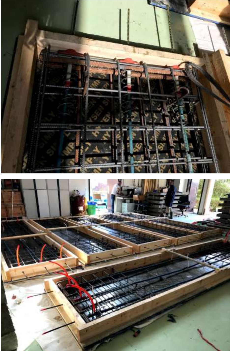
Figure 4-13 Shows the hooks' location in the UBSR 1 specimen (top) and the six one-way post-tension slab specimens before concrete casting (bottom)
