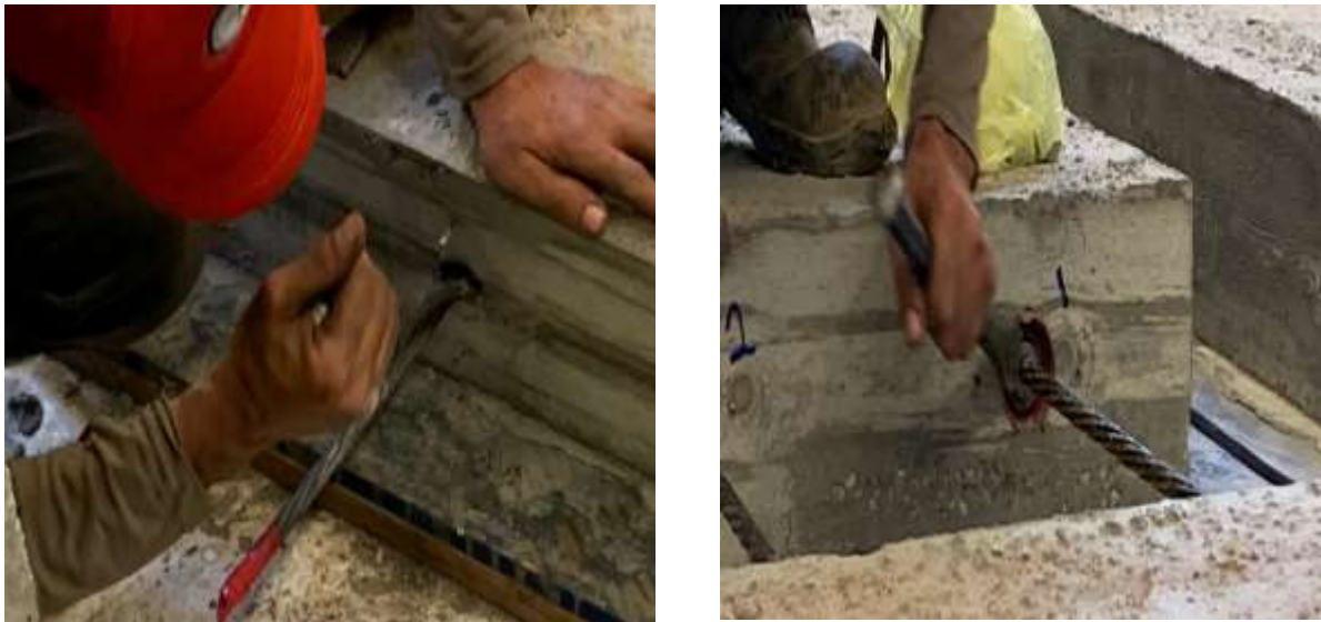
Figure 4-19 Cleaning process for the bonded tendon anchor opening from concrete mortar (left) and wedges installation into the bonded and the unbonded anchors (right)
