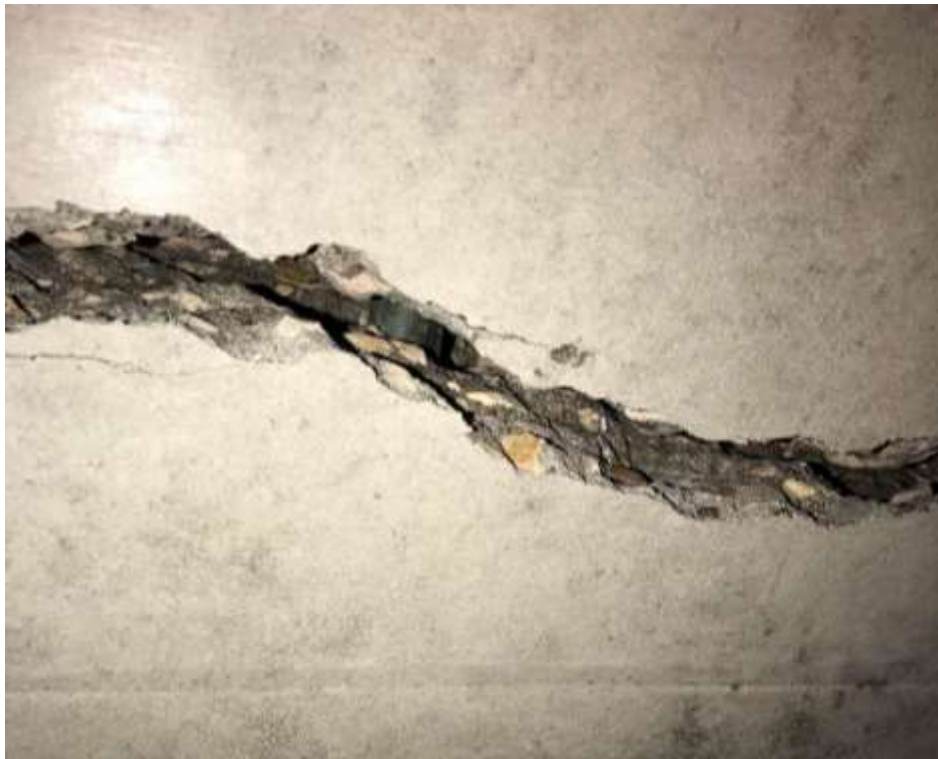
Figure 5-11 UBS1 failure mode (top) and concrete bottom surface crack showing the prestressing tendon (bottom)
