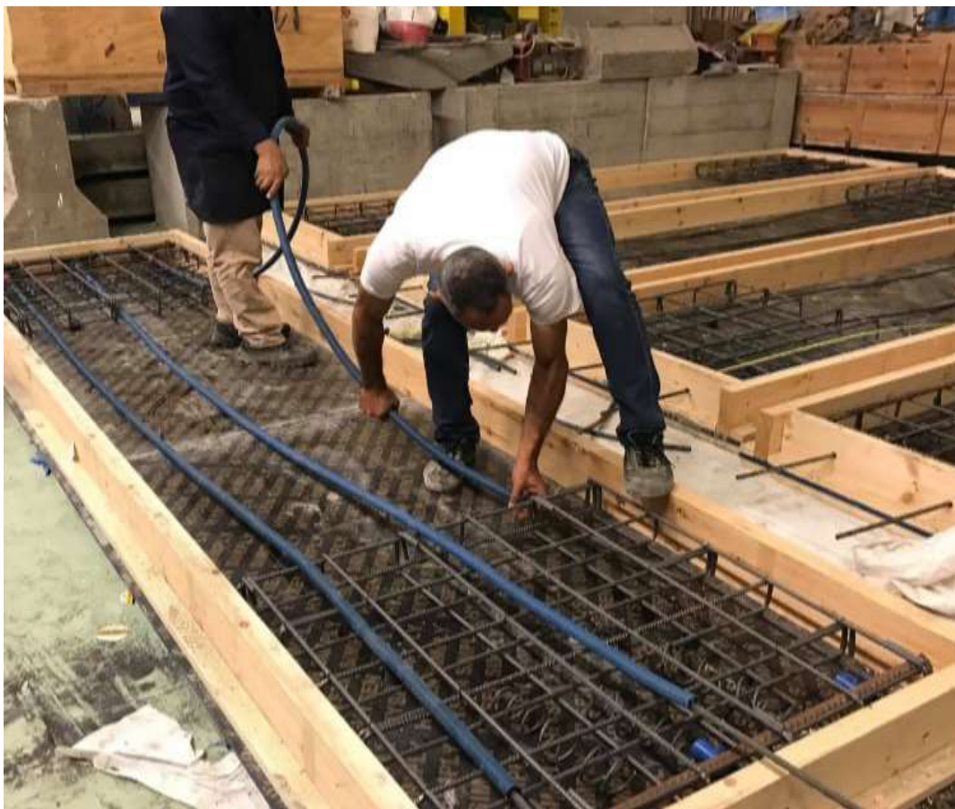
Figure 4-8 Unbonded anchors installed in their designed spots with the spiral stirrups and the two bars of diameter 25mm are shown after fixation in their final position (top) and the bonded tendons inserted in the corrugated plastic duct are fixed with the designed profile in their designed locations (bottom)
