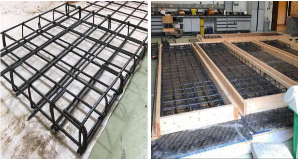
Figure 4-3 Stirrups of bars no.10 mm in the two dimensions forming a cage (left) and detailing of reinforcement of the two unbonded slabs with non-prestressing steel reinforcement (right)
