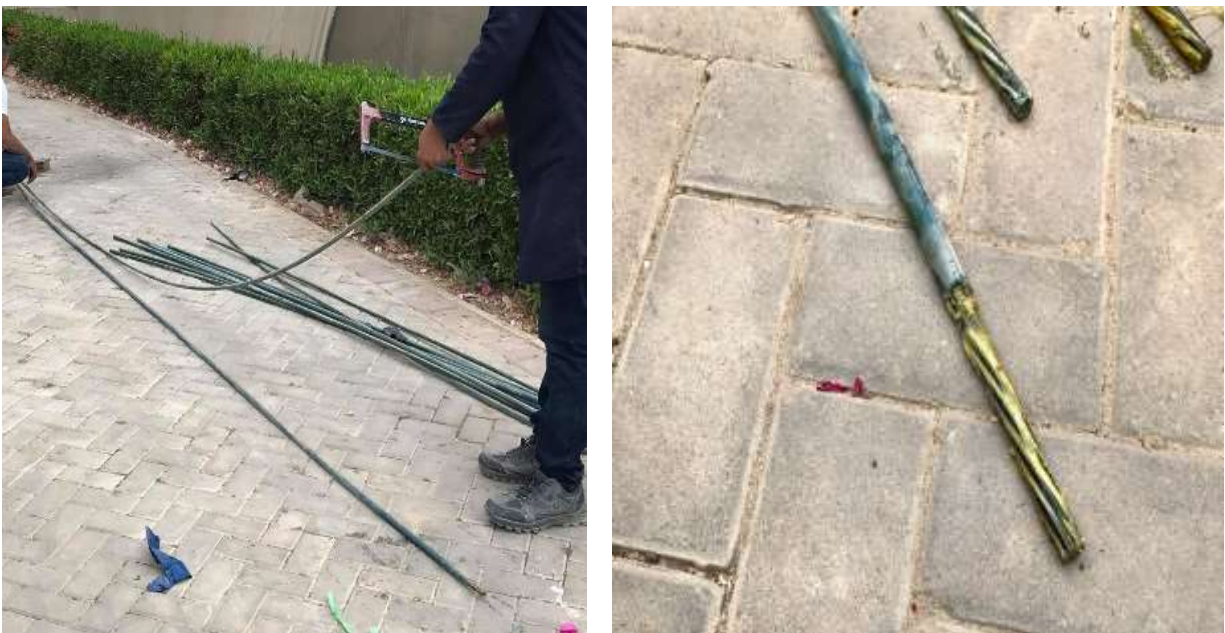
Figure 4-7 Prestressing cables are cut down to 5.0m each (left) and the unbonded tendons covered with grease and extruded plastic sheathing (right)
